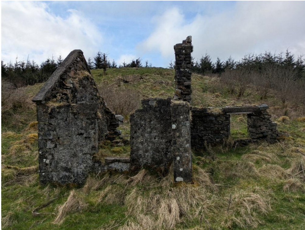
Plate 14-15 Southeast elevation of vernacular building (CH12) within T06 hardstand and turbine base, facing northwest
