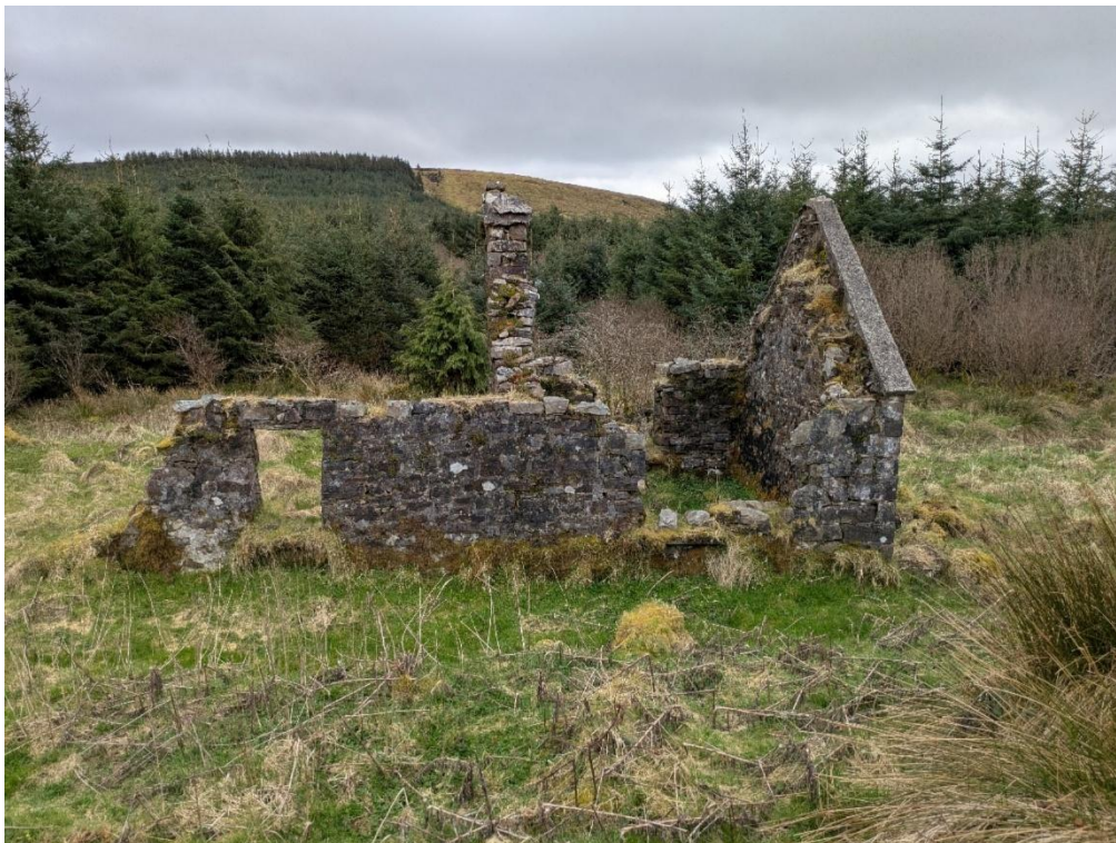
Plate 14-16 Northeast elevation of vernacular building (CH12) within T06 hardstand and turbine base, facing southeast
